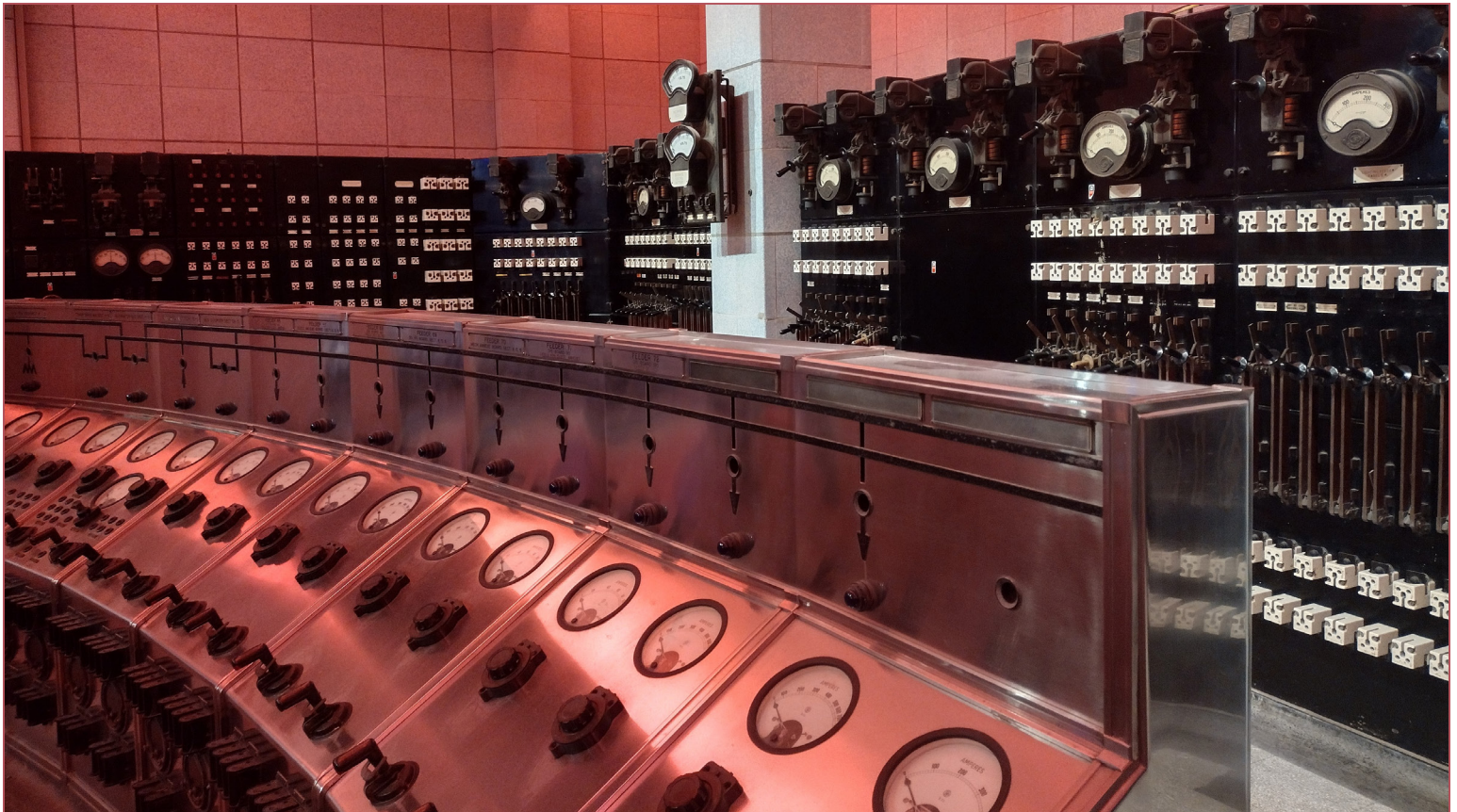
Part of the controls of the Battersea Power Plant in London, England restored and open to the public.
