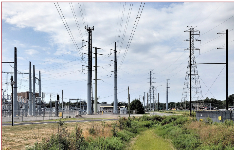
Newark to Trenton Fast Trolley former right of way. The Metuchen Switching Station visible at left.
